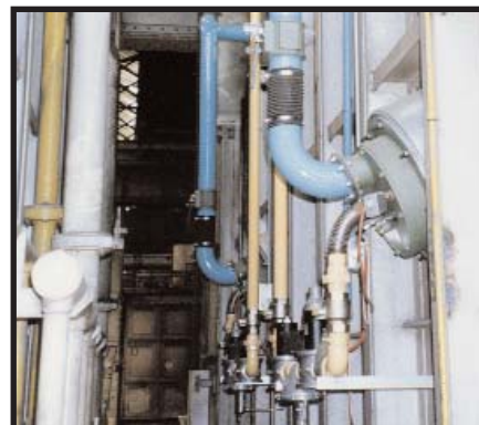
Car Bottom Furnace
